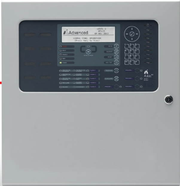
Redundant Panel Takes Control
