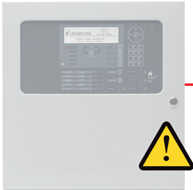
Main Panel in Fault
